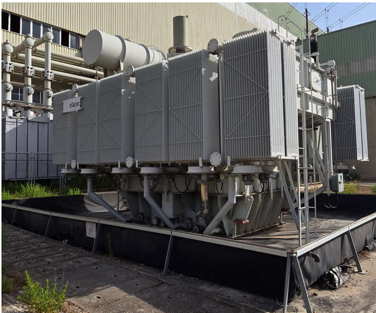
Figure 15: overview of spare transformer
