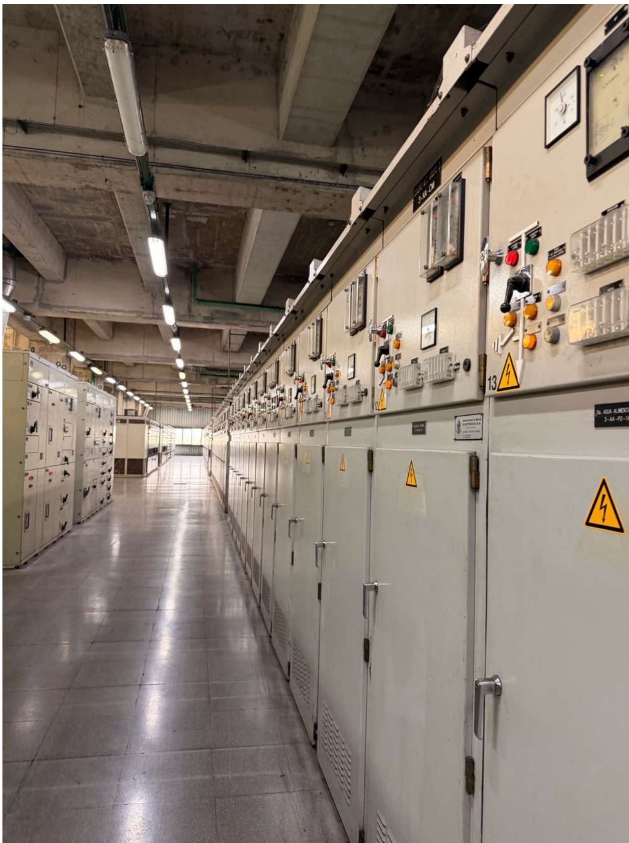
Figure 16: detail of MCC Group4
