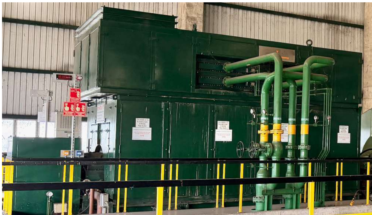
Figure 12: overview of the generator with its exciter.
