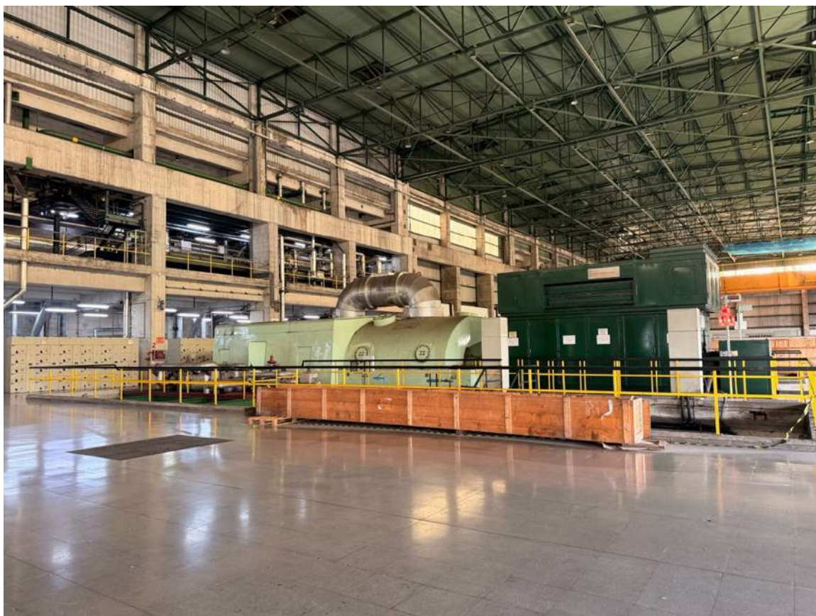
Figure 5: overview of the steam turbine Unit3
