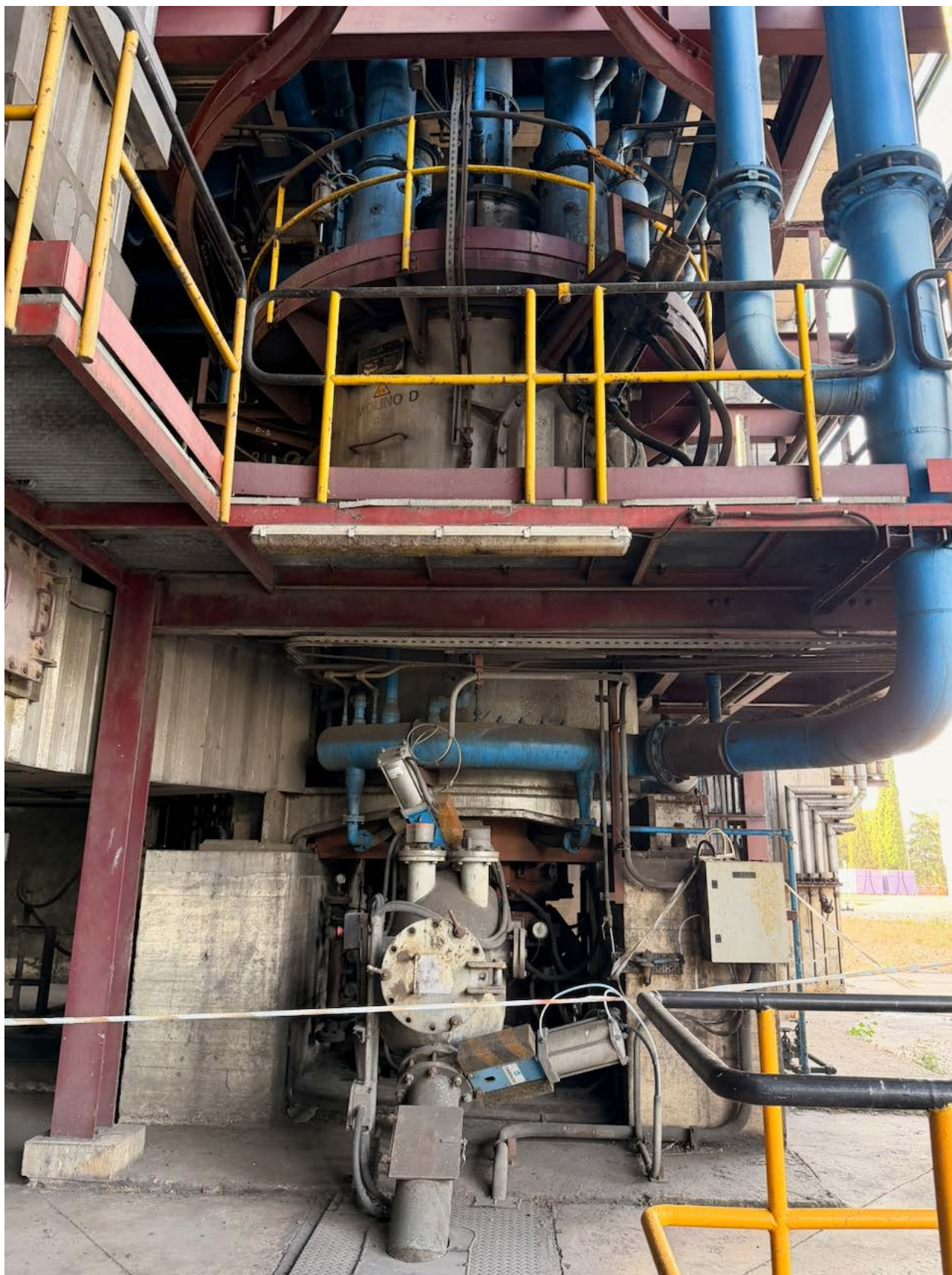
Figure 24: coal mill. Perfectly cleaned.
