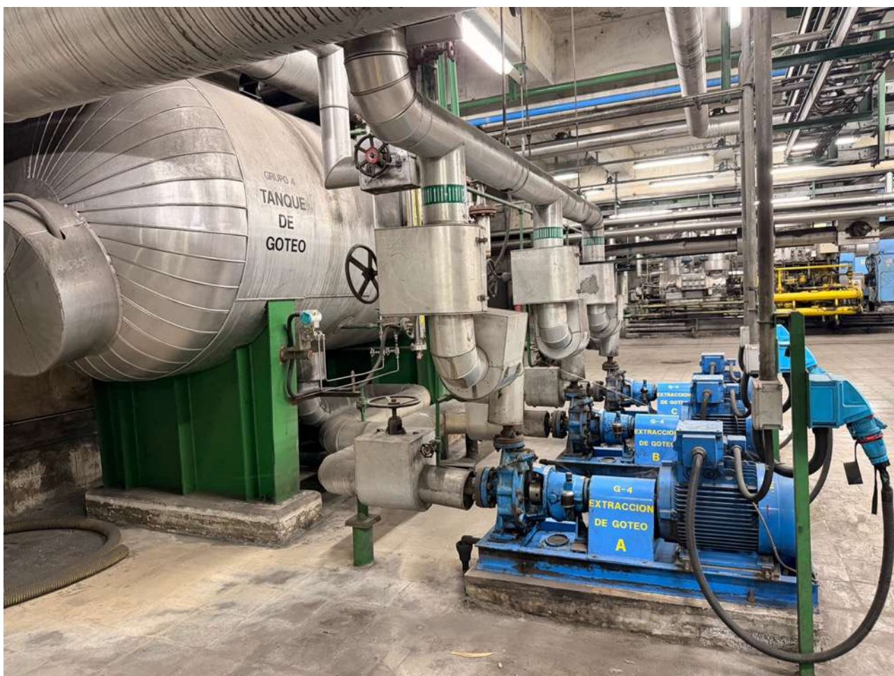
Figure 11: overview of drain tank
