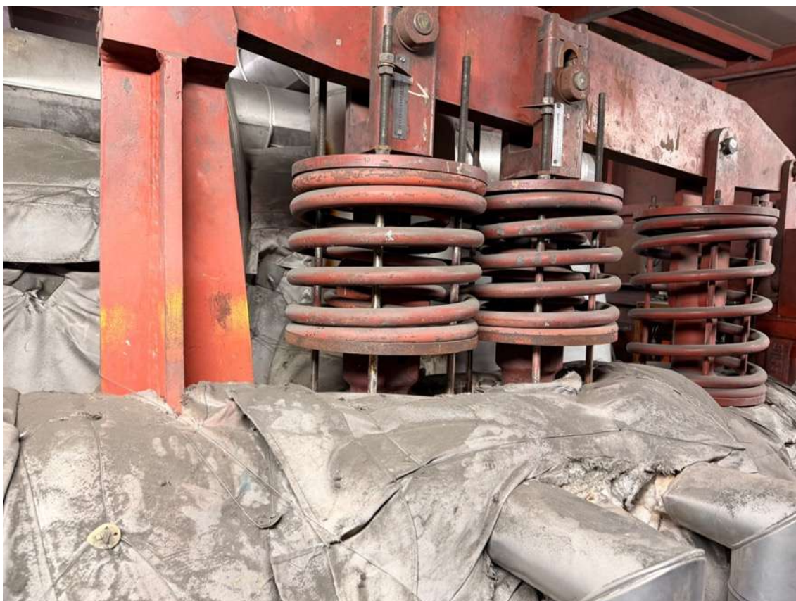
Figure 7: detail of the HP turbine, Unit3
