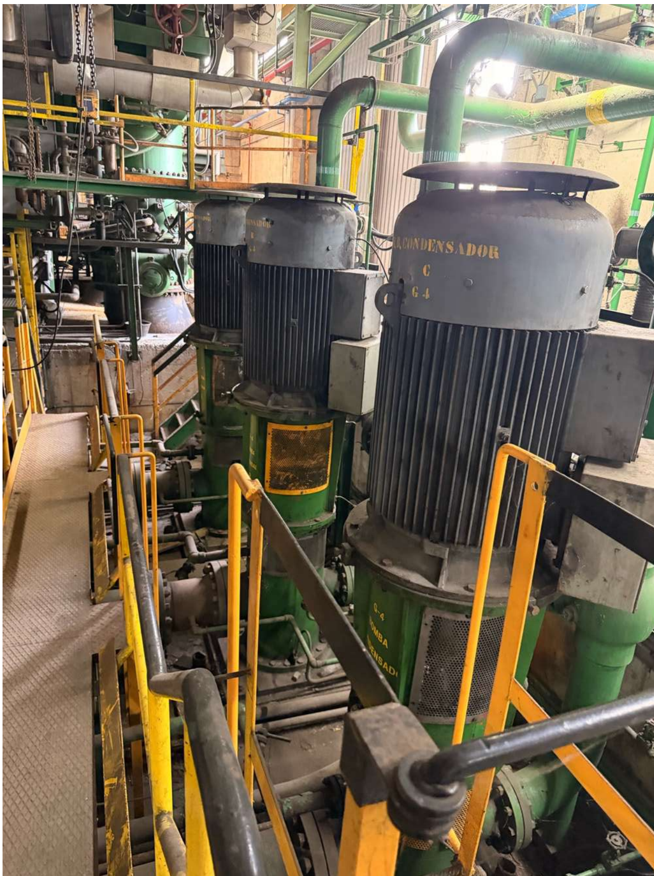
Figure 10: detail of condensate pumps
