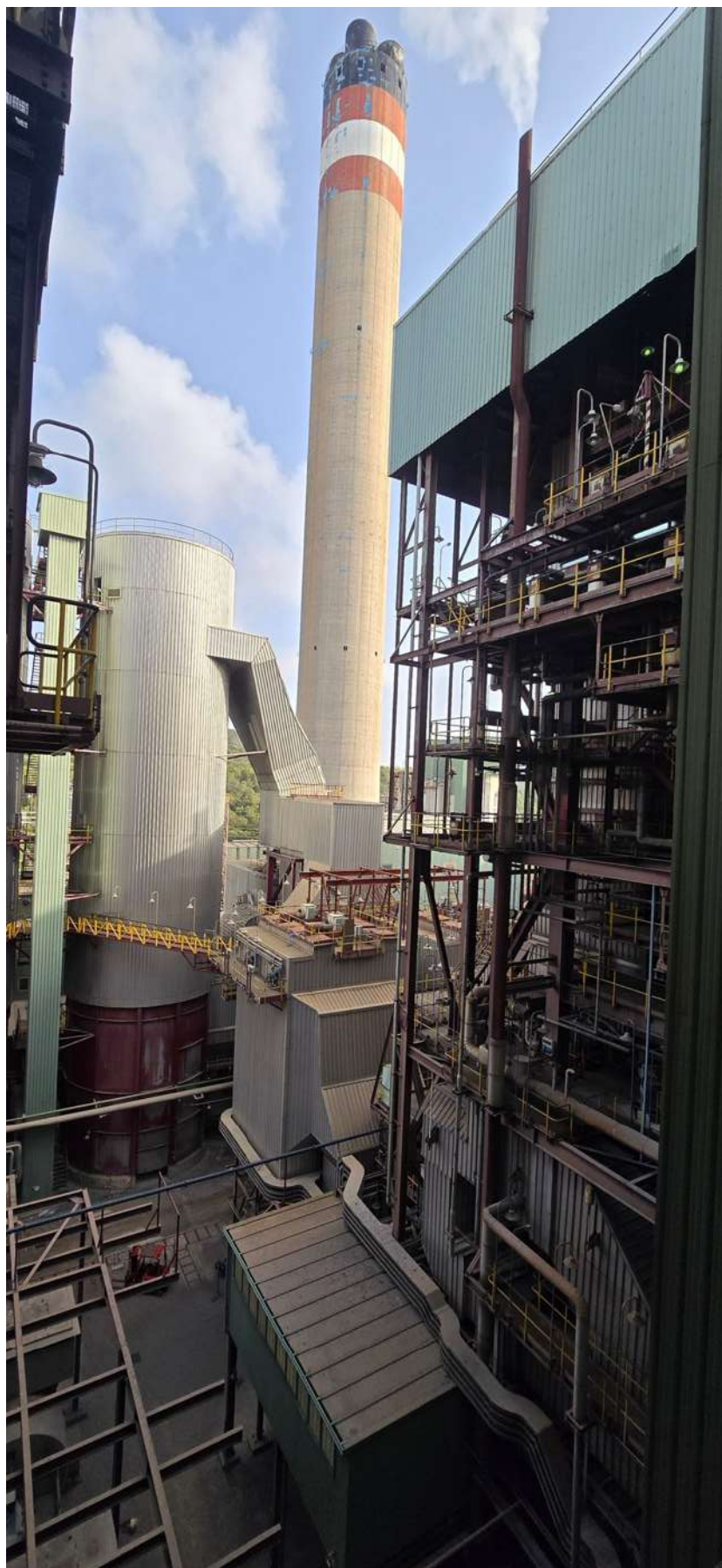
Figure 22: side view of the boiler Unit3.
