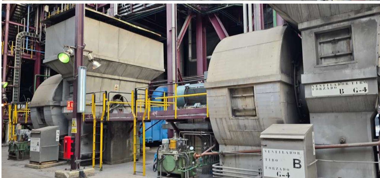
Figure 23: the sooth blowers are installed below the boiler, the fresh air blowers on the sides
