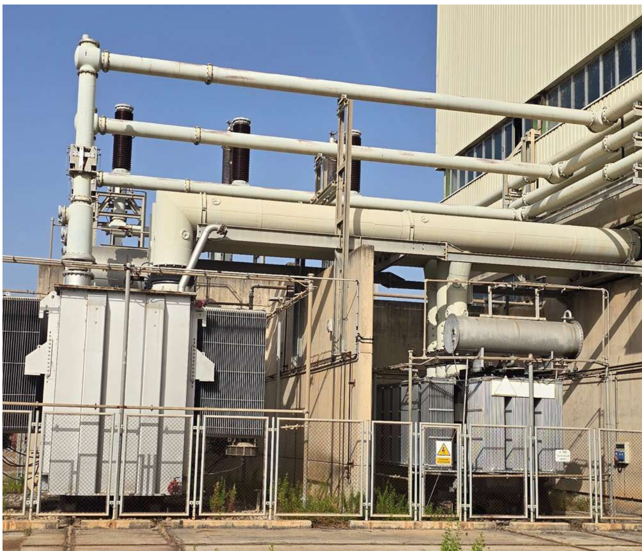
Figure 13: overview of transformers
