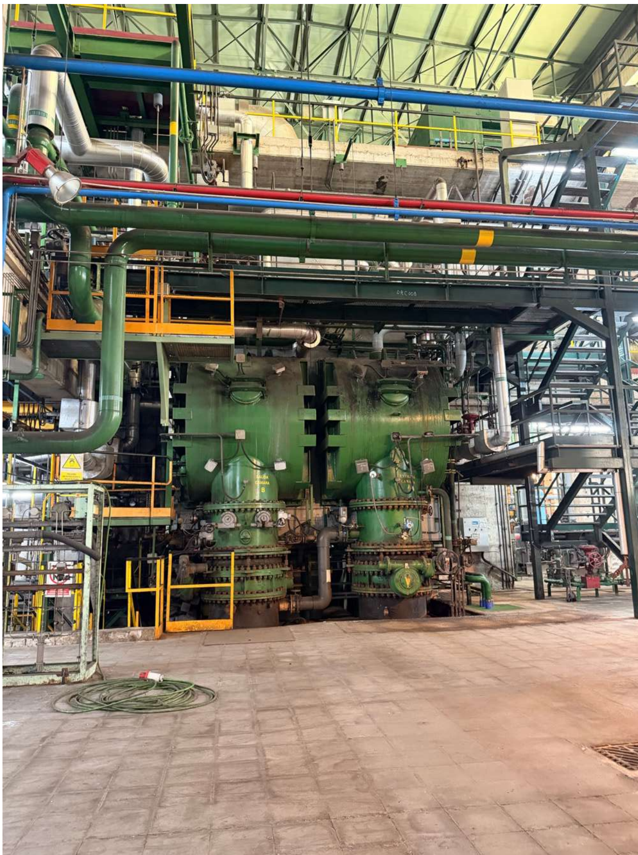
Figure 9: overview of the condenser
