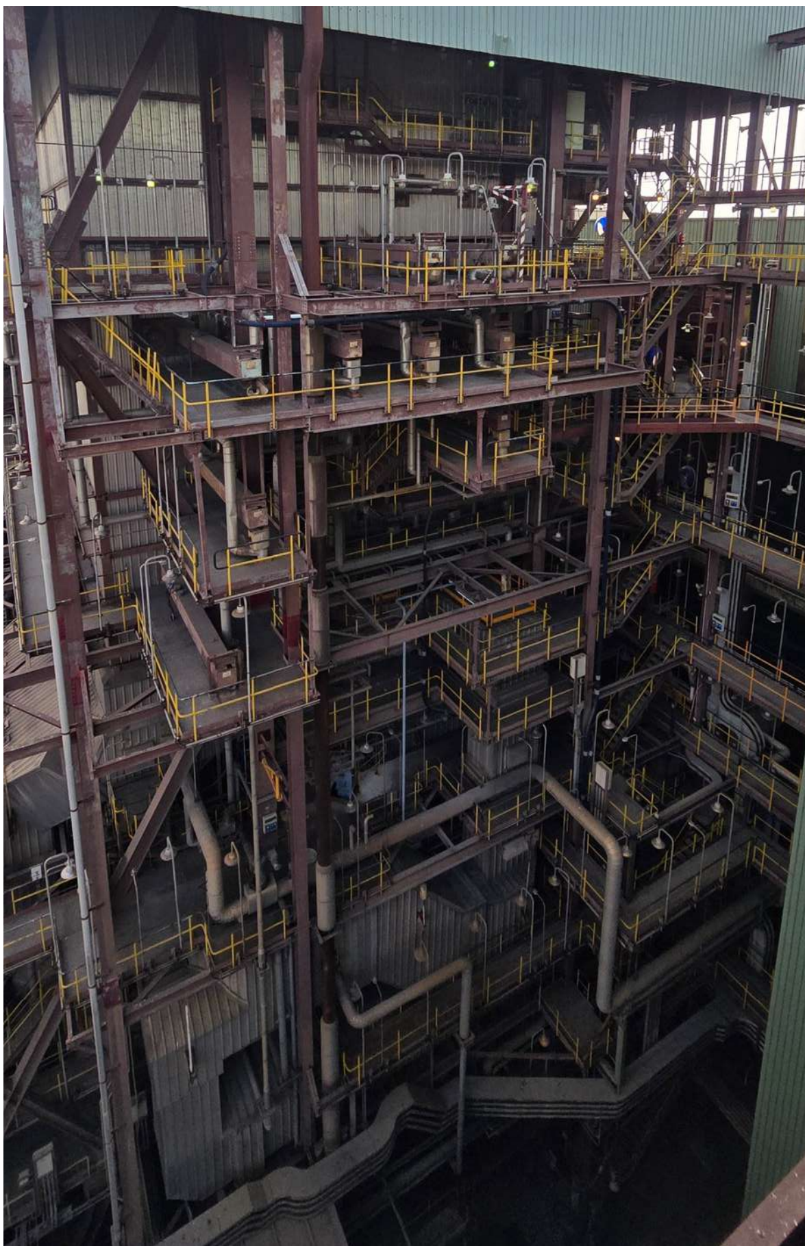
Figure 21: side view of the boiler Unit4
