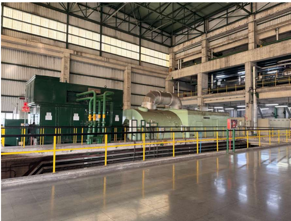
Figure 6: overview of the steam turbine Unit4
