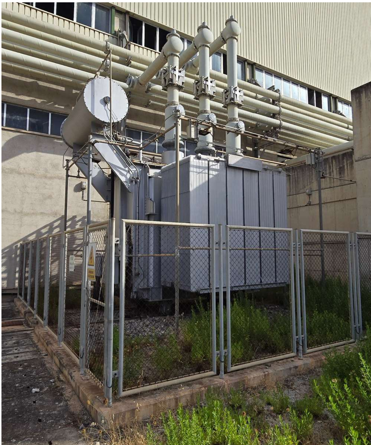
Figure 14: overview of transformers
