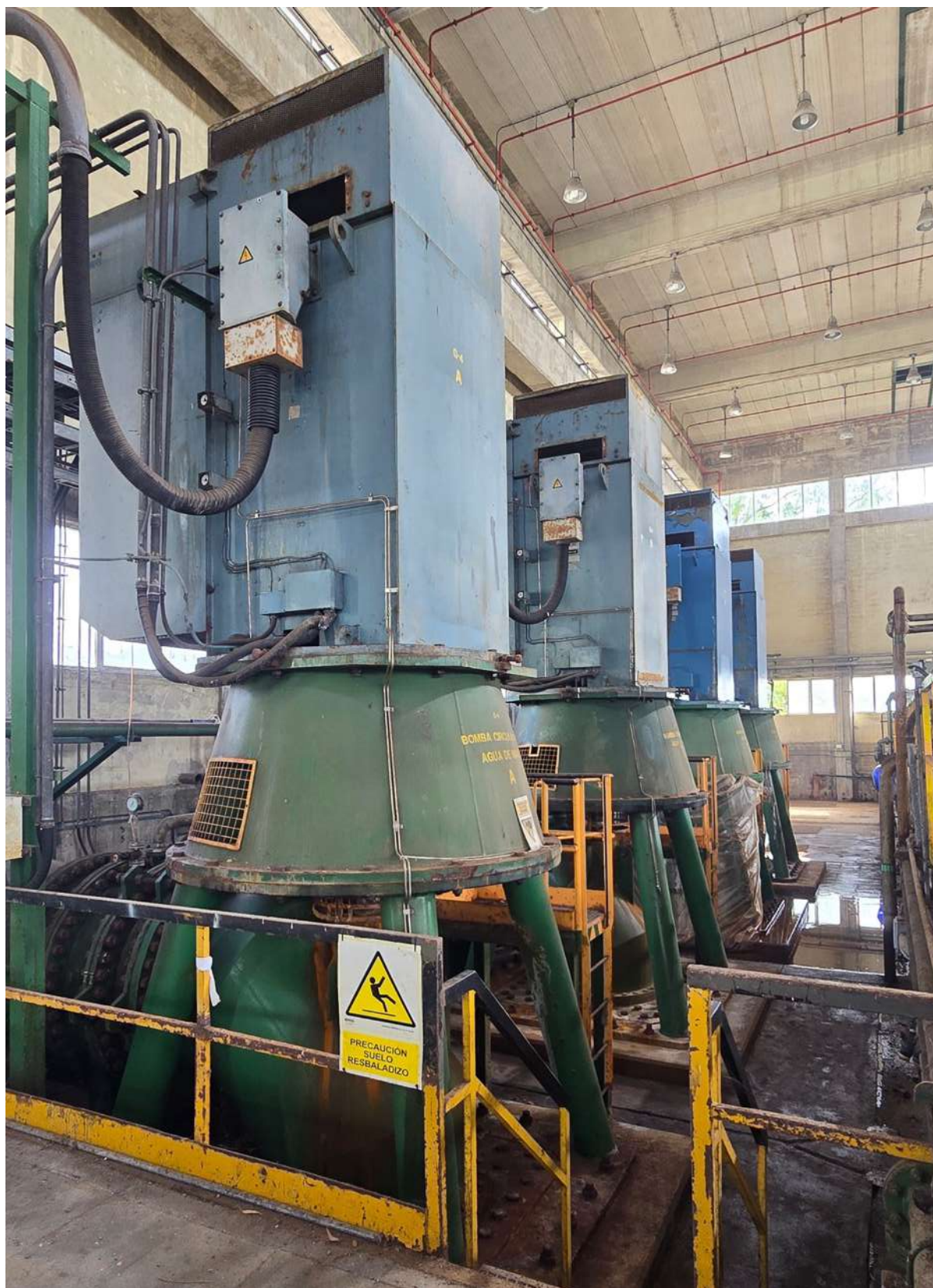
Figure 17: Seawater cooling water pumps
